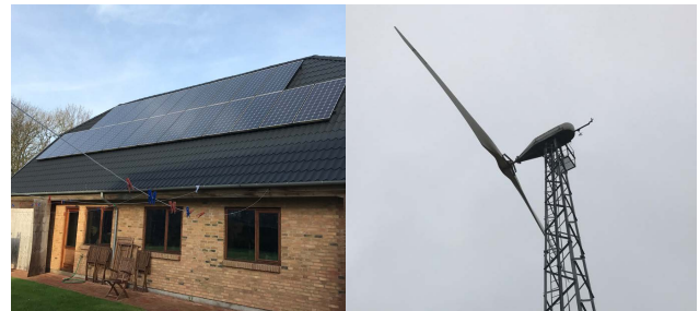
Figure 1. PV installation in H3 (left) and wind turbine in H4 (right).
