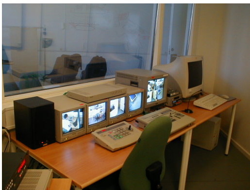
Figure 4. Control room: equipment for operating the motorized video cameras in the subject room.
